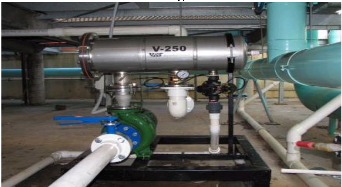
Cooling Tower Water Filtration
