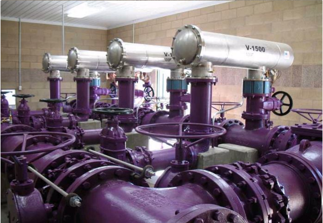
Irrigation Water Filtration
