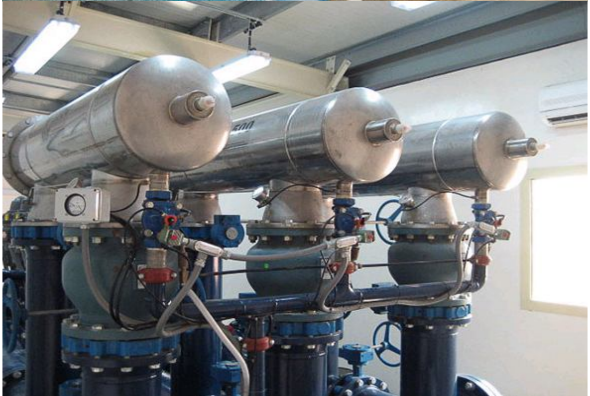
Irrigation Pond Water Filtration
