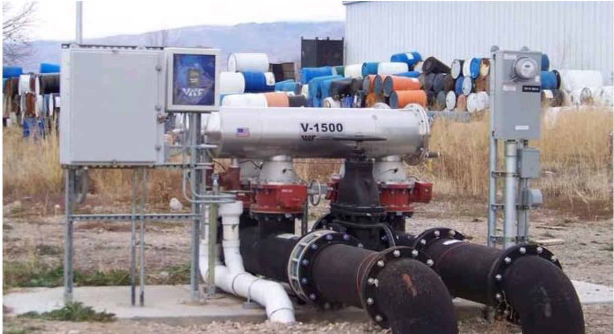
Filter Skid With Bypass Manifold
