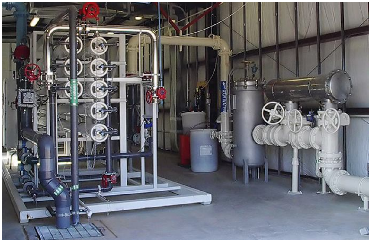
Filtration of Reverse Osmosis-Pre
