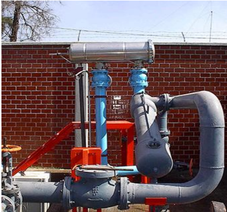
Centrifugal Sand Separators-Cooling Tower Filtration
